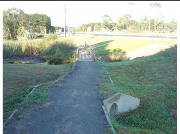
A short piece of the path to the recreation reserve (at the crossing of Lavers-Hill Cobden Rd) is missing and needs to be constructed.
