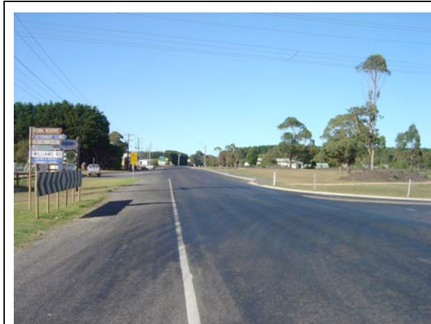
Some scope exists for improving on-road conditions for cyclists on the Lavers Hill – Cobden Rd, painting edge lines (to create a sealed shoulder for cycling).
