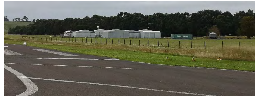
Figure 12 Runway edge and end lighting
