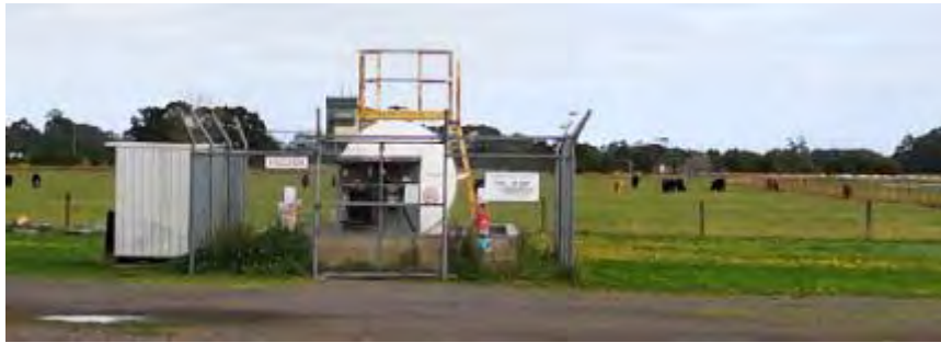
Figure 9 Fuel (Avgas) facility
