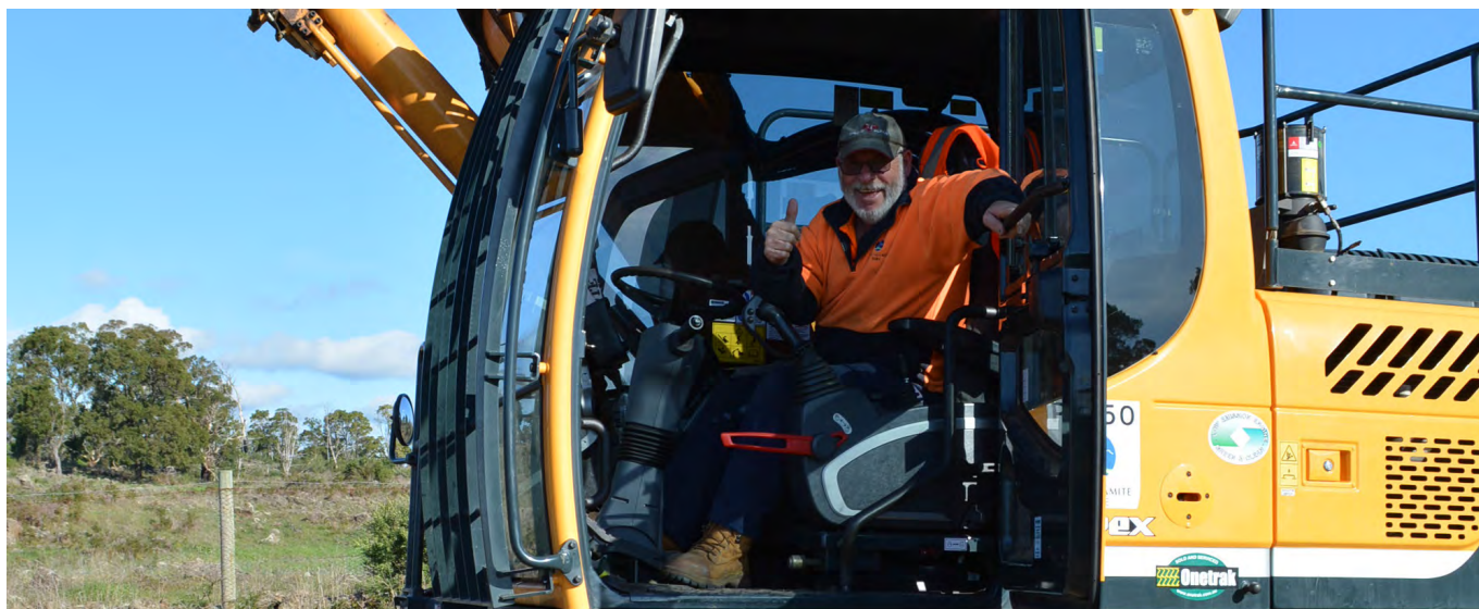
Operator Vinnie Carter in the new wheeled excavator carrying out drainage works at Hawkes Nest Road in Pomoroneit
