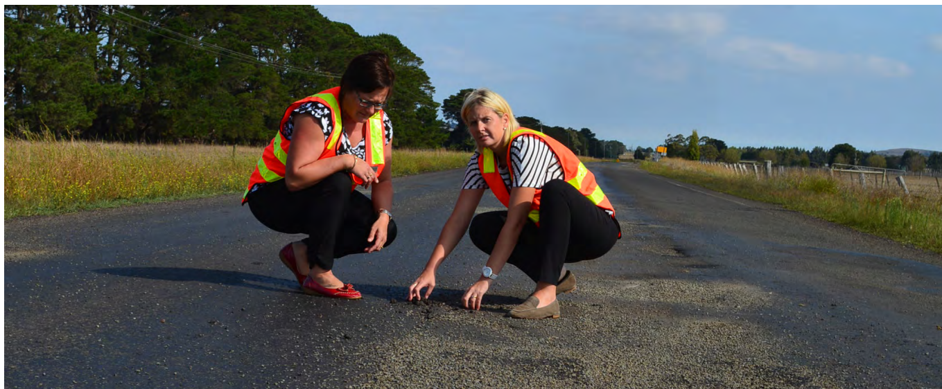
Mayor Jo Beard and Director Works and Services Brooke Love inspect the poor condition of a State Government managed road
