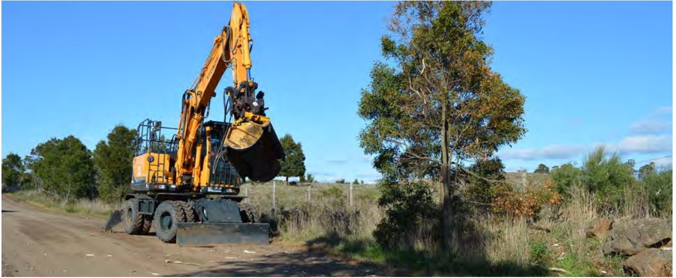
The wheeled excavator carries out drainage clearance works at Hawkes Nest Road in Pombooneit
