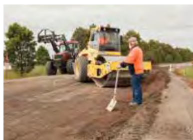
Photos from far left: Foxhow Road prior to widening by VicRoads; Shire roadworks
